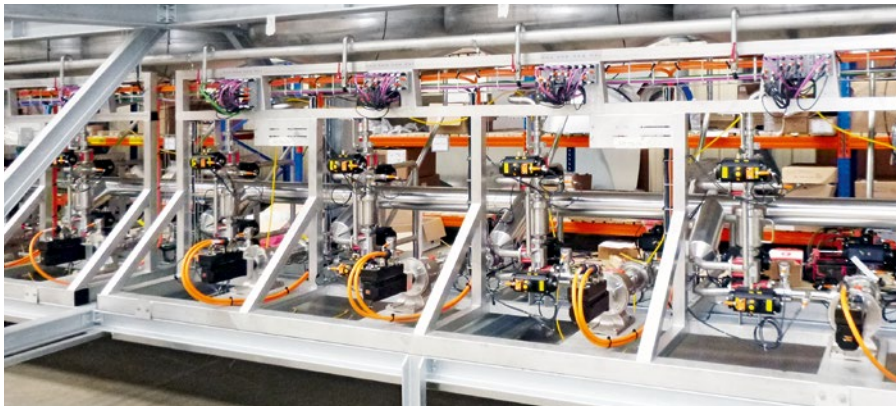
Decentralized motion control with B&R's ACOPOSmotor servo actuators allows Dynavia to offer modular machinery with reduced cabling and simplified architectures – giving its customers the flexibility to adapt to future demands.
