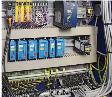
The compact B&R components fit nicely into the control cabinet of the trimmer.
